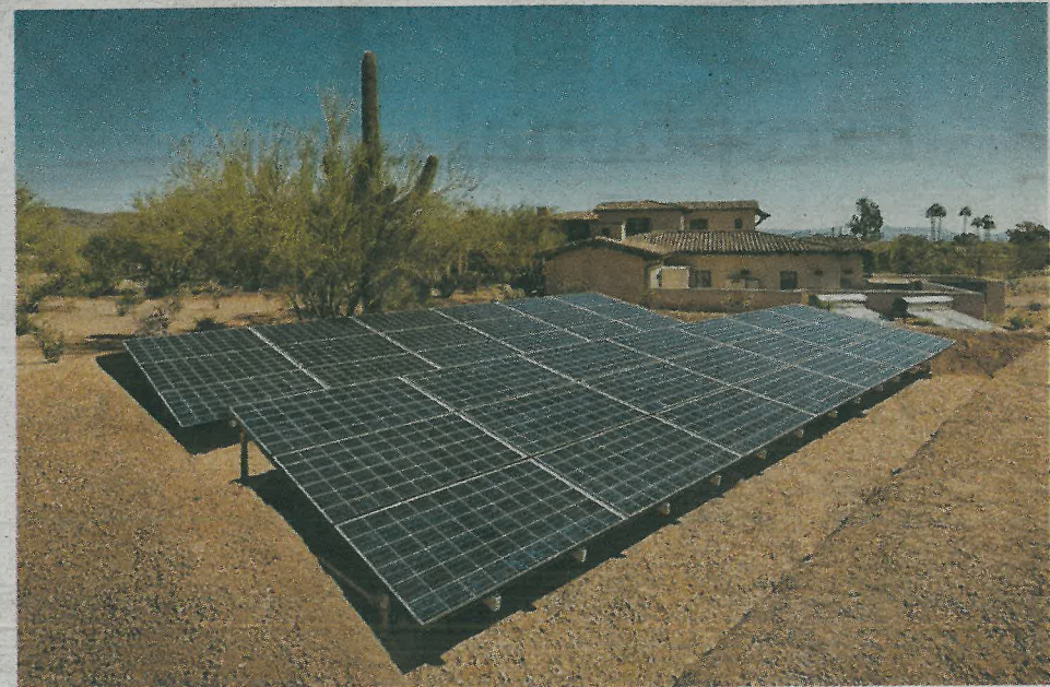
This photovoltaic array is set away from the home rather than on the roof. The solar cells are used to generate electricity for the home, casita and guesthouse.
